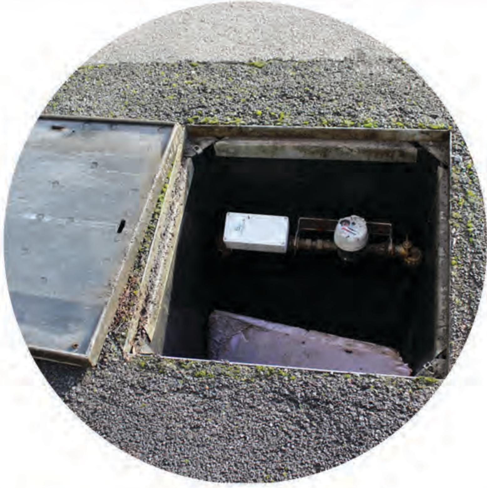
A STREGA Smart-Valve installed below ground surface into a chamber for automatic pipe flushing
