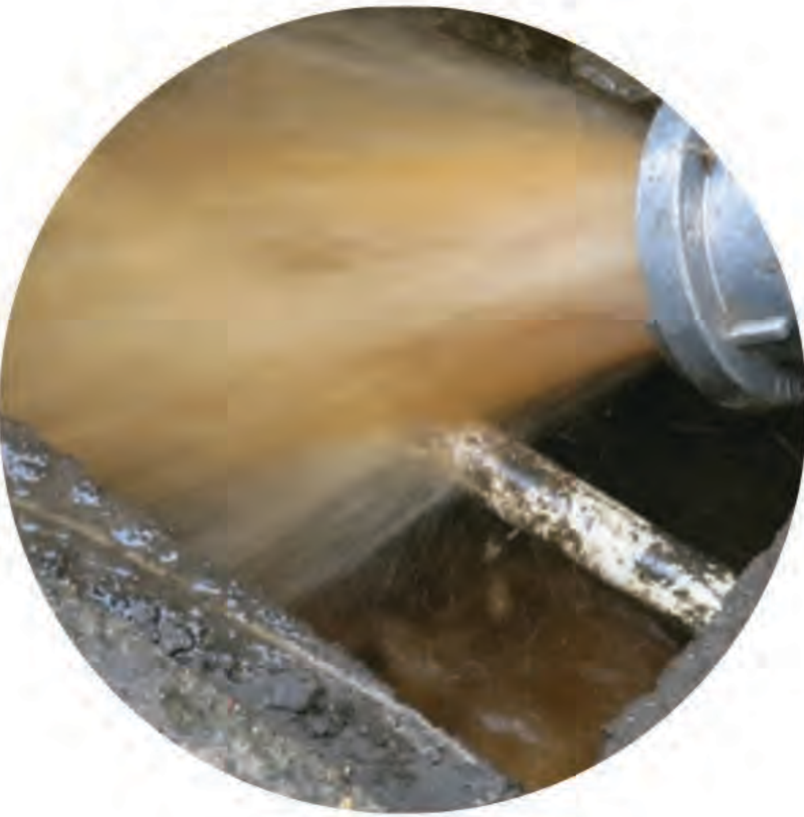
The automatic flushing is carried out without human presence and at preprogrammed intervals by performing the opening and closing operation to drain the water to the river or the rainwater network.
