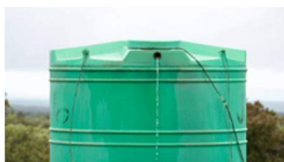
Tank level Monitoring
