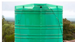
Tank Level Monitoring
